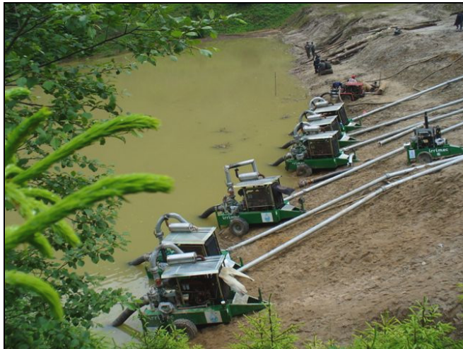
Fig. 6. Mitigation measures in order to evacuate the excess water from the top of the Tarnicioara tailing dam
