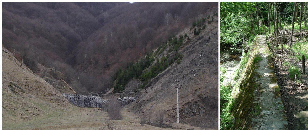
Fig. 7. Torrent control works: right tributary of Iara River (left); Brăzești Valley (right)
