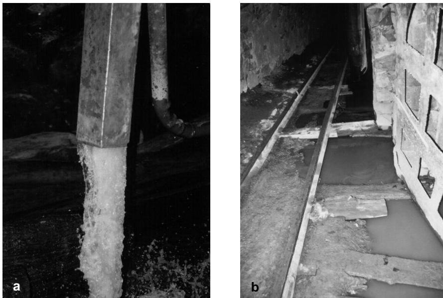
Fig. 4. Acidic mine water management: a – underground water pumped to the main adit, b – water transported by the underground channel
