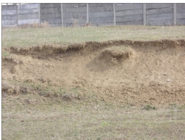
Fig. 1. Landslide in the proximity of the compressor station
