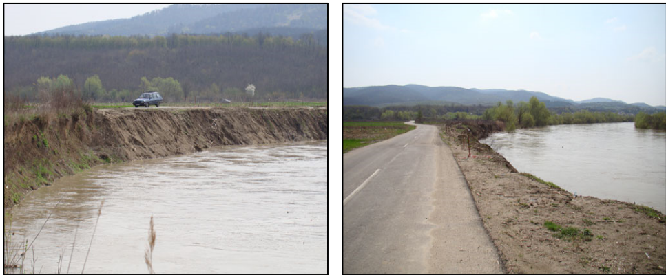
Fig. 10. Shore erosion during the 2010 flood, near Ulmeni
