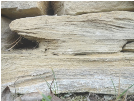
Fig. 4. Delamination and granular disintegration.
