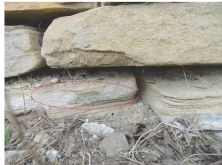
Fig. 5. White efflorescence caused by the dissolution of calcium carbonate.
