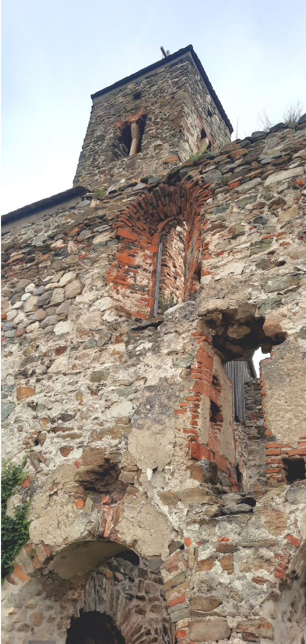
Fig. 10. Details of the consolidation with concrete beams, view from the south, 2023. (photo: I. Rus-Cacovean).
